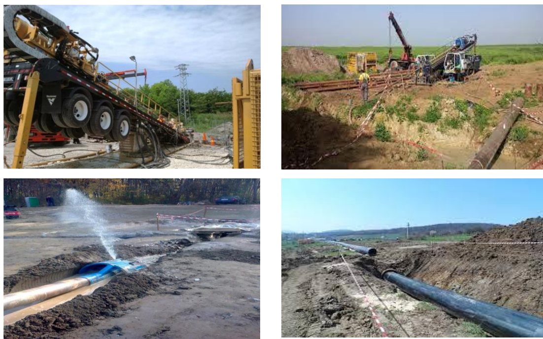
Fig. 1-4 Horizontal directional drilling equipment and drilling works during the undercrossing of the Danube River [7]
