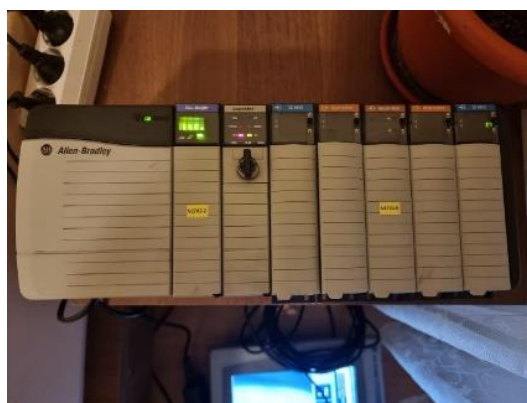
Figure 2. Allen Bradley 1756 PLC with L61 processor
