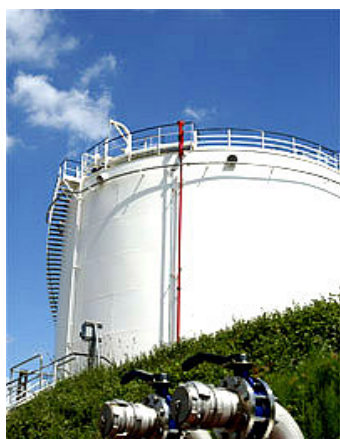
Fig.4. A hydrocarbon storage at the petroleum depot in le mans, with fire extinguishing system in the foreground.
