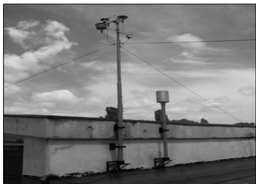
Fig. 1.a. System for environmental monitoring of metrology type AWS / EV from the aculty I.S.B. Bucharest [3]
