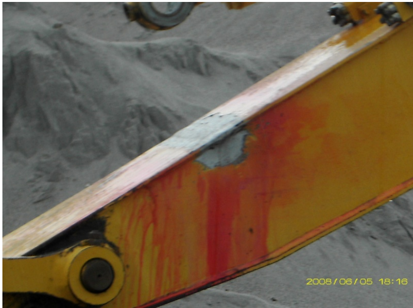
Fig.5. Arm repaired by welding after grinding the seams and penetrant testing examination
