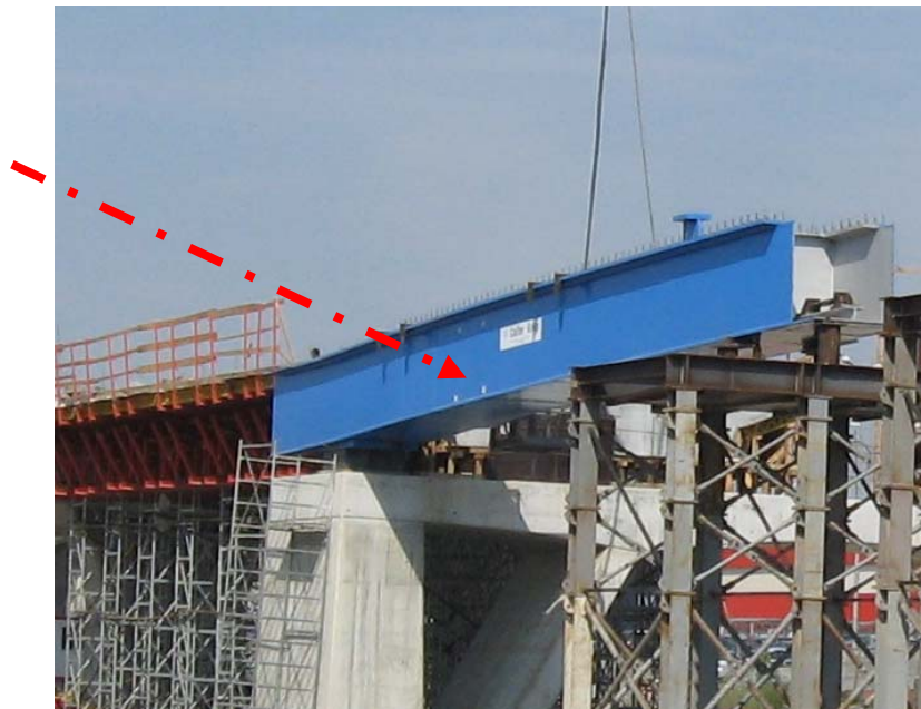
Fig.6. Placing the section No.1 of the beam longitudinal on the support device
