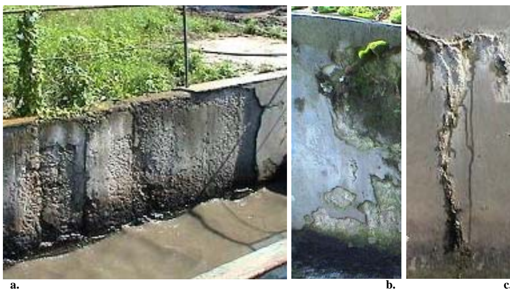
Fig. 2. Surface-aerated basin. a.- sidewalls deteriorated by bio-corrosion; b., c.- details
