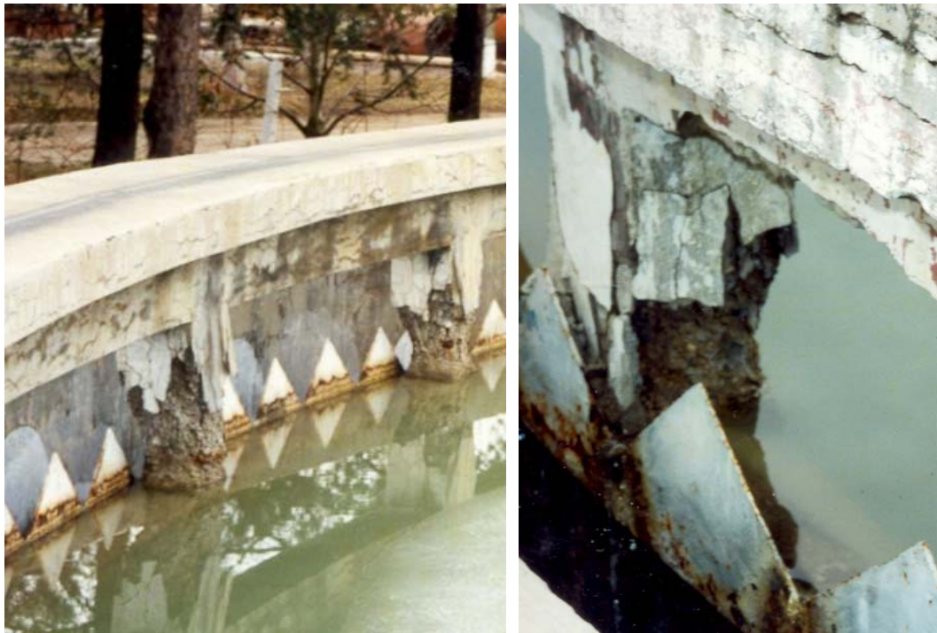
a. Fig. 1. Radial settler D 25 m. a.- Cracks in the crain-beam and columns due to sulphatic corrosion and level variations; b.- Detail b.
