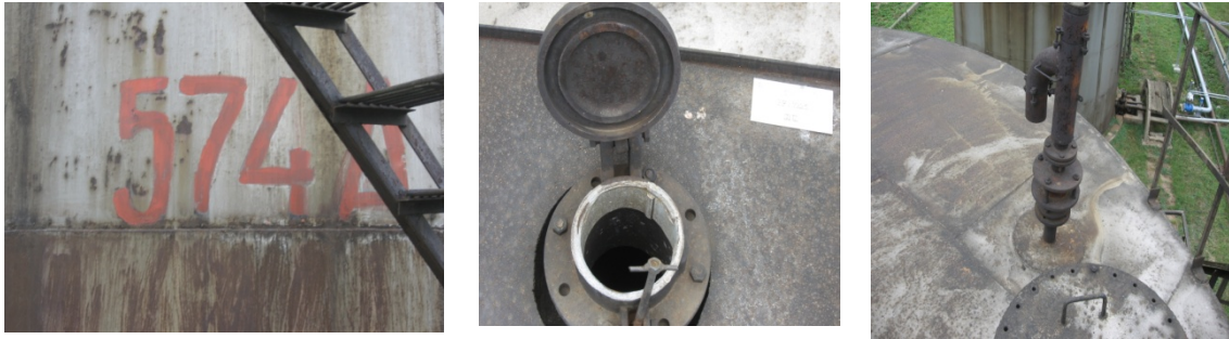
Fig. 5. The 574A tank, having the respiratory equipment outdated and unworkable, with the discharge of emissions into the atmosphere through the manhole
