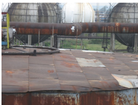
Fig. 4. The TK28A, TK28B tanks physical status
