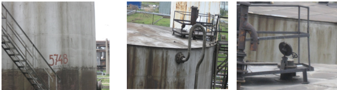
Fig. 6. The 574B tank, having the respiratory equipment outdated and unworkable, with the discharge of emissions into the atmosphere through the manhole
