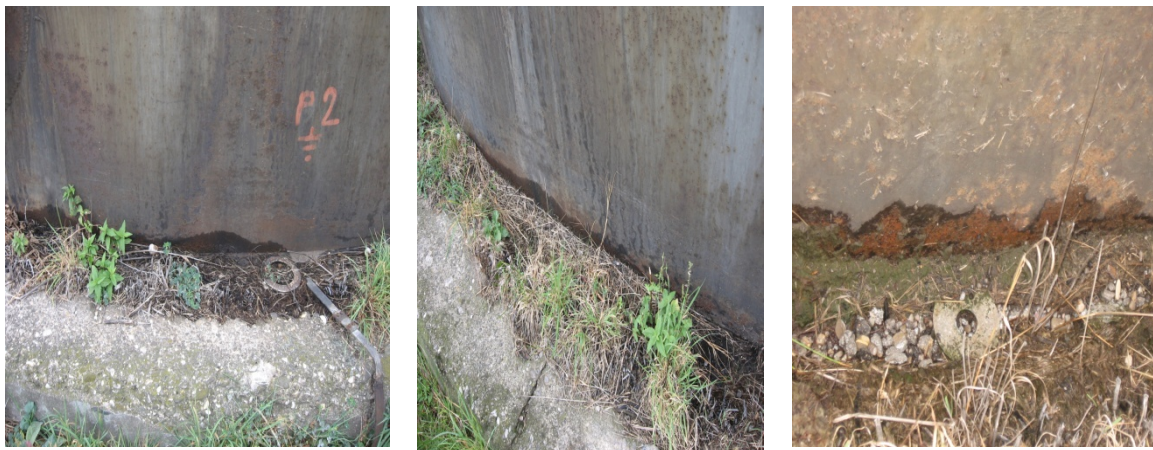
Fig. 9. The tank 587 presents an advanced corrosion at the bottom-mantle junction
