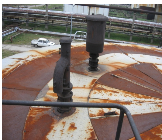
Fig. 1. The respiratory safety equipment, not working, completely rusty
