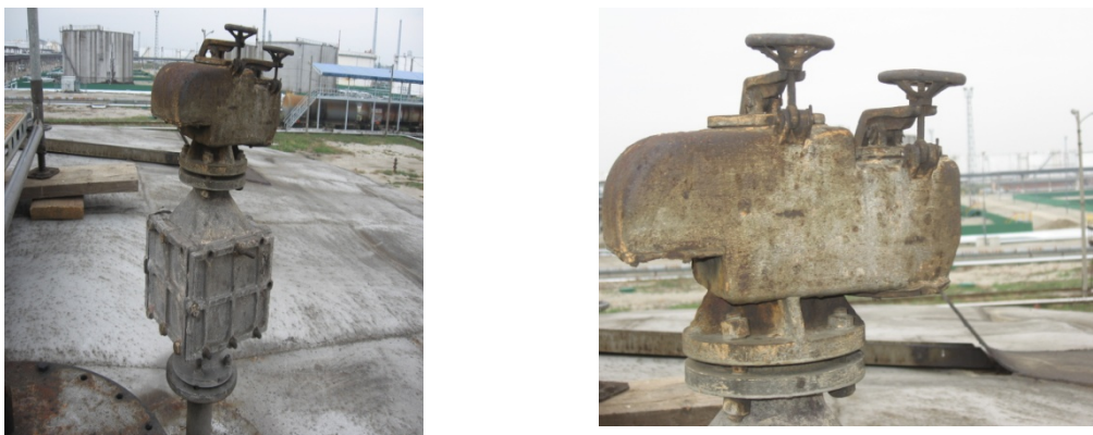
Fig. 8. The 587 tank, provided with a safety respiratory equipment outdated and unworkable, with arrester flame and mechanical breathing valve
