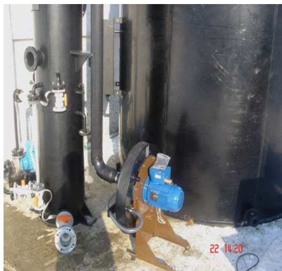
Detail to show up humidifier, fan and water recirculation pump
