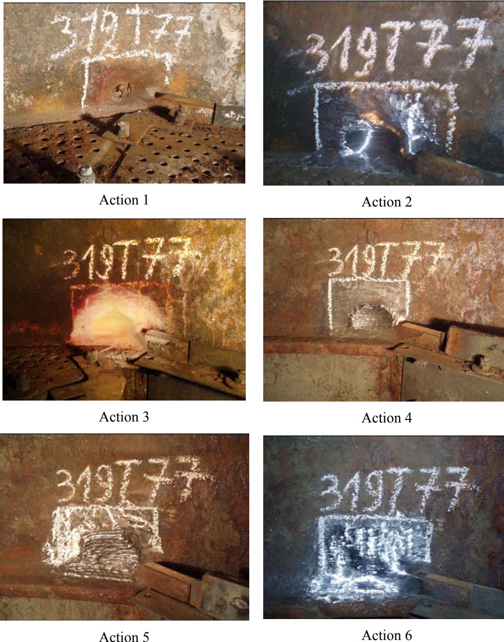
Fig. 4. Short visual review of aspects related to the repair welding technology for a pressure equipment damaged due to ongoing processes induced by technologic fluids (courtesy of Subsidiary ROMAG PROD from RAAN)
