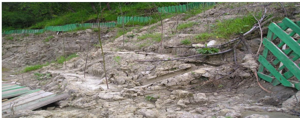
Fig. 10. Embankments and berms on the western side of the lake – F1 and F2 drilling area – image taken on May 23 rd , 2014
