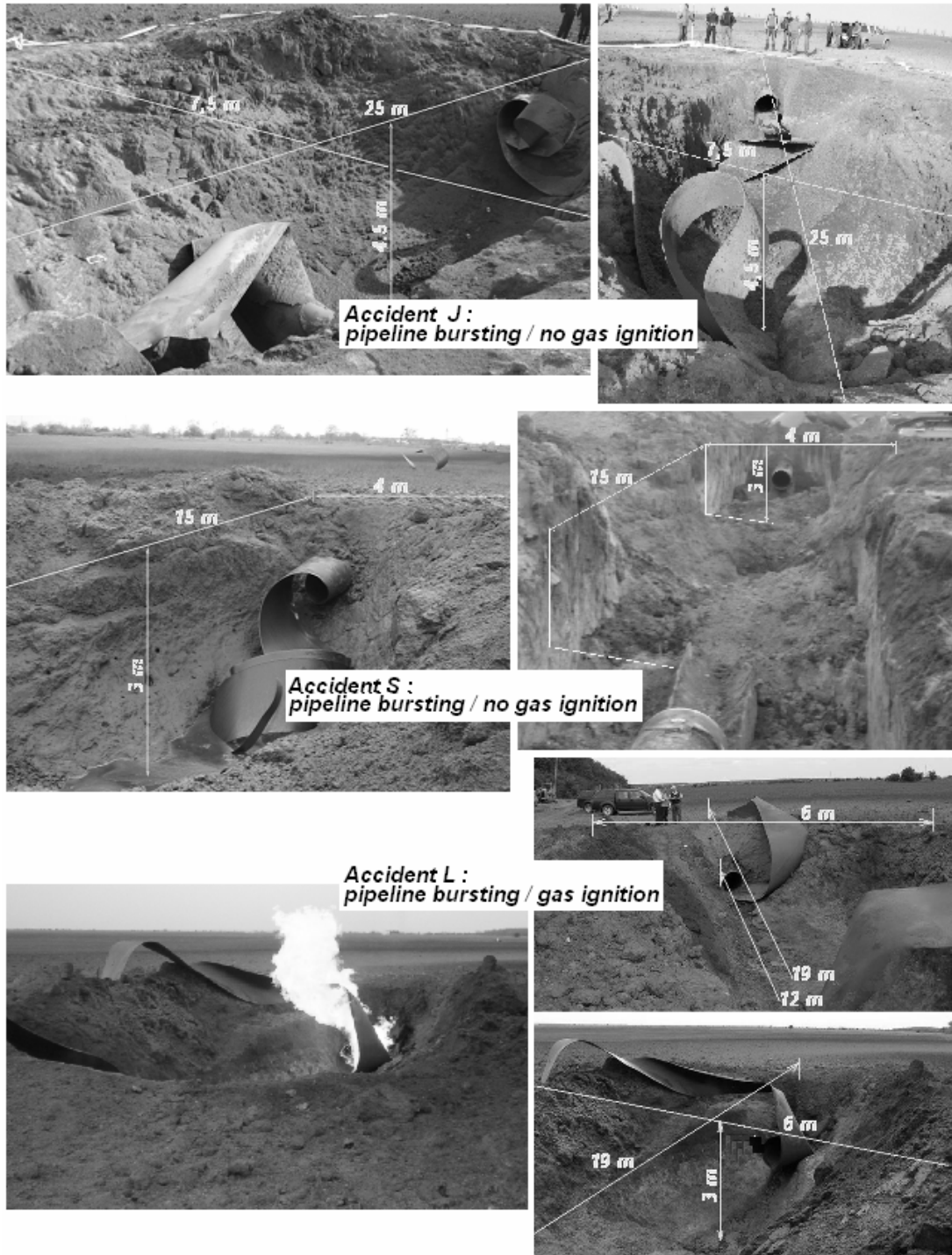
Fig. 2. Technical accidents produced due to lamination-like flaws of the pipes the natural gas transmission pipelines are made of
