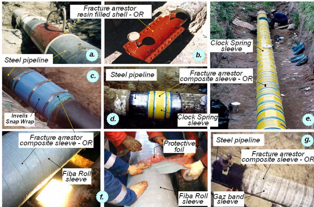
Fig. 2. Types of fracture arrestors and their coding a, b fracture arrestors resin wrap, code OR – A1.B1.C1.D1 or OR – A1.B2.C1.D1; c, d. fracture arrestor composite wrap, code OR – A1.B1.C3.D5 or OR – A1.B2.C3.D5 ; e, f, g. fracture arrestor composite wrap, code OR – A2.B1.C3.D5 or OR – A2.B2.C3.D5
