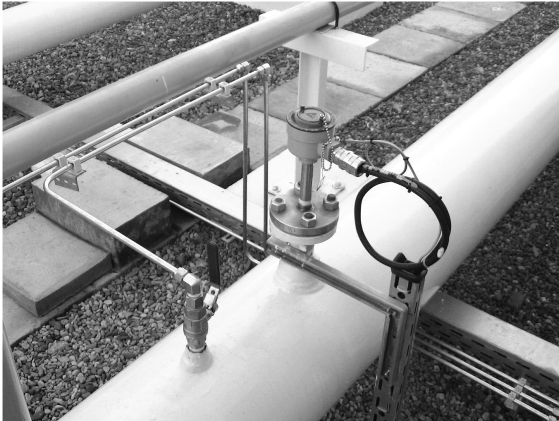
Fig. 6. Gas flowrate metering from a Romanian compressor station.
