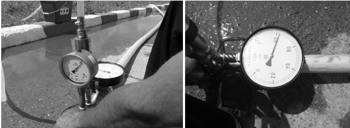
Fig. 4. Inlet pressure and vacuum gauges.
