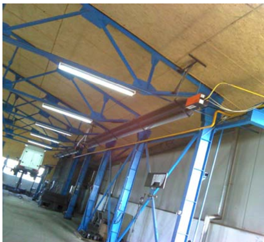
Fig. 2. The hall and the radiant tube where the thermovision measuring has been performed
