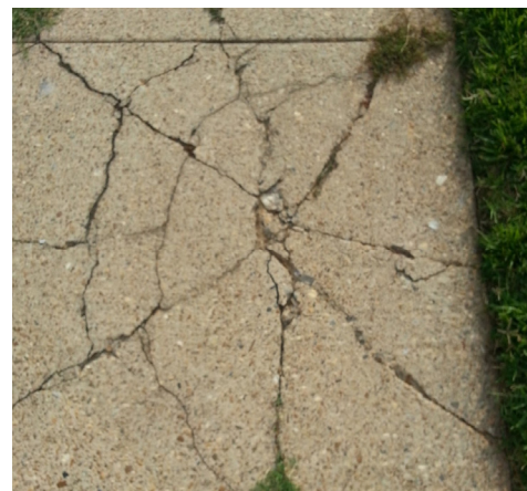
Fig. 15. Radial cracks, and not only, in a pavement [12]
