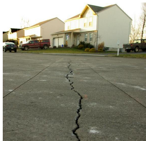
Fig. 10. Crack in asphalt [9]
