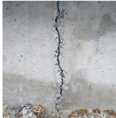
Fig. 8. Crack in concrete foundation [7]
