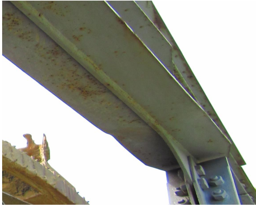
Fig. 3. Major deformation zone that appeared in the HL beam.
