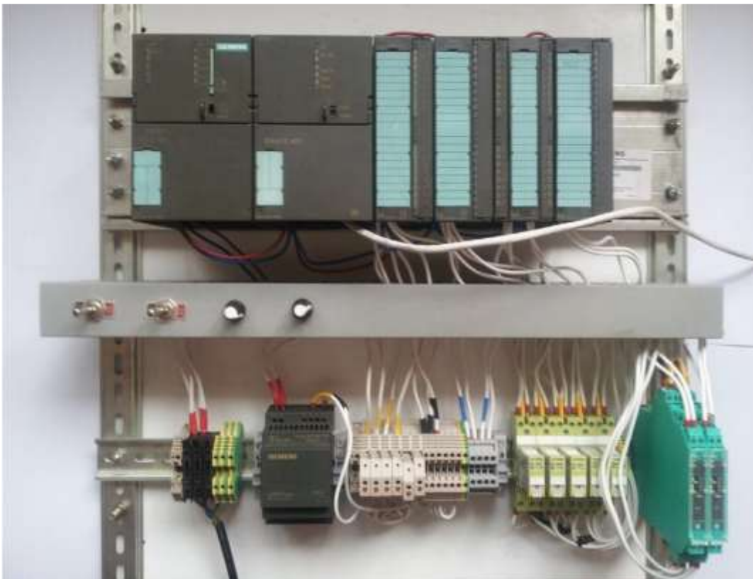
Fig. 2. PLC connections to the laboratory plant.
