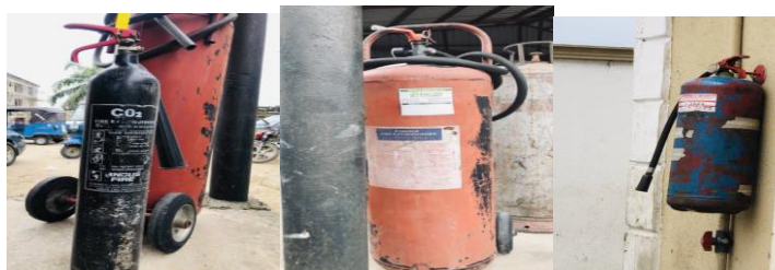
Plate 1. Visible fire extinguishers
